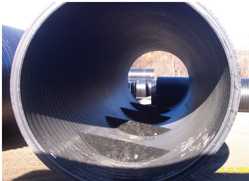
Baffles are placed off center from the invert or flowline of the culvert and remain on one side of the culvert and do not alternate.
